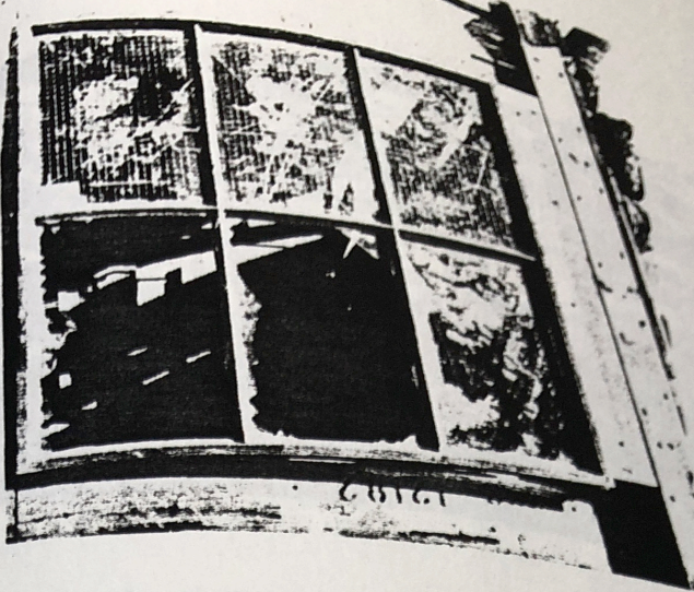
Figure 3 - Shattered Window Panes in "Cabin" at 6800 ft Equivalent Distance (see Section 6)
